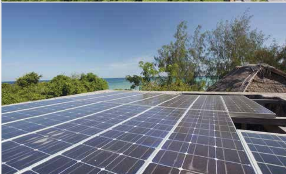
CHICOP employs the exclusive use of renewable energy with these solar panels powering the facility (Photo courtesy CHICOP)
