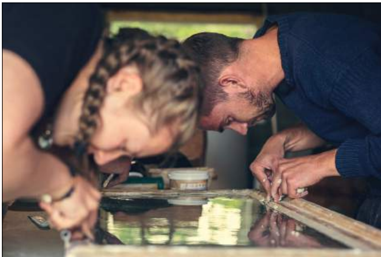
Figure 8.9 Course in window restoration in Å in Lofoten, organised under the auspices of the National Trust of Norway.
